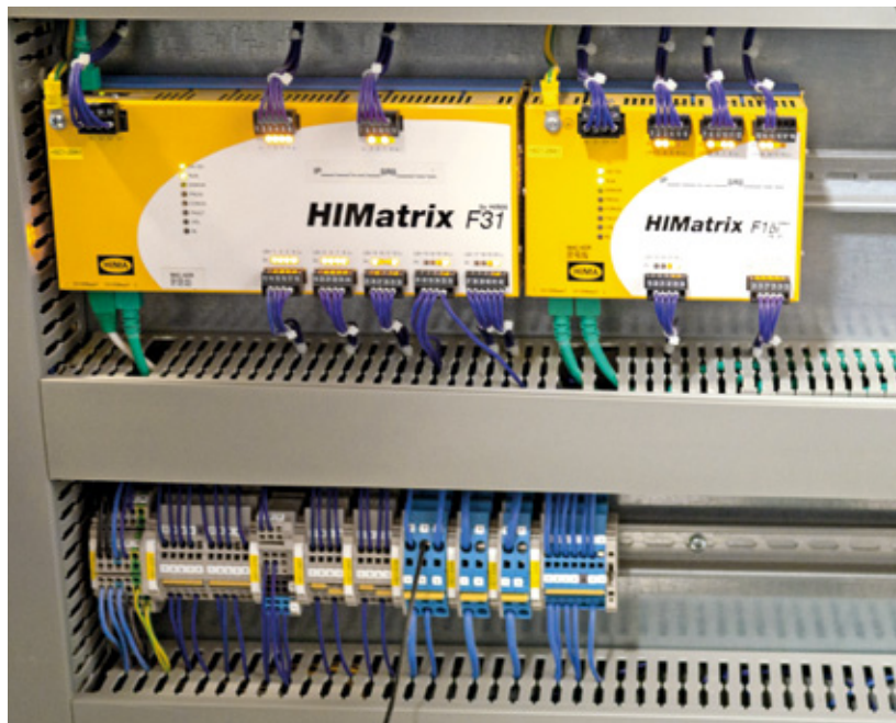
The HIMatrix in the control cabinet coordinates the other controllers in the rides
